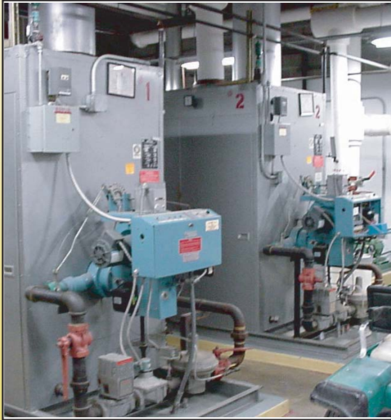
Boiler: B&W D-type rated at 100psig, equipped with low Nox burner
