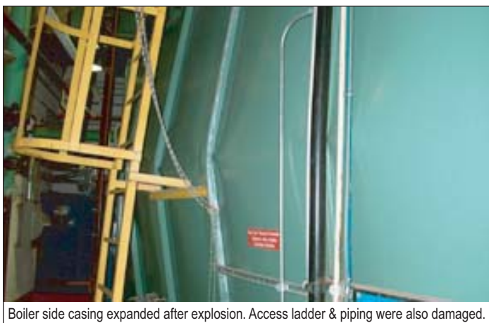
Boiler side casing expanded after explosion. Access ladder & piping were also damaged.
