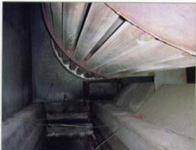
Repair damage such as refractory breakdown or tube failures and ruptures as required.
