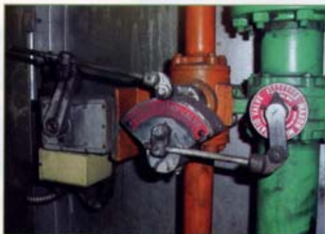
Experienced burner-tuning technicians should set fuel-air ratios.
