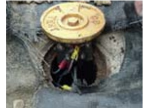
Access point for easily testing cathodic protection.
