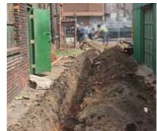
Replacing damaged piping can be expensive and time consuming.
